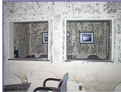
Photo courtesy of OSHA. This picture shows actual disaster site work conditions and may not illustrate proper safety and health procedures.
